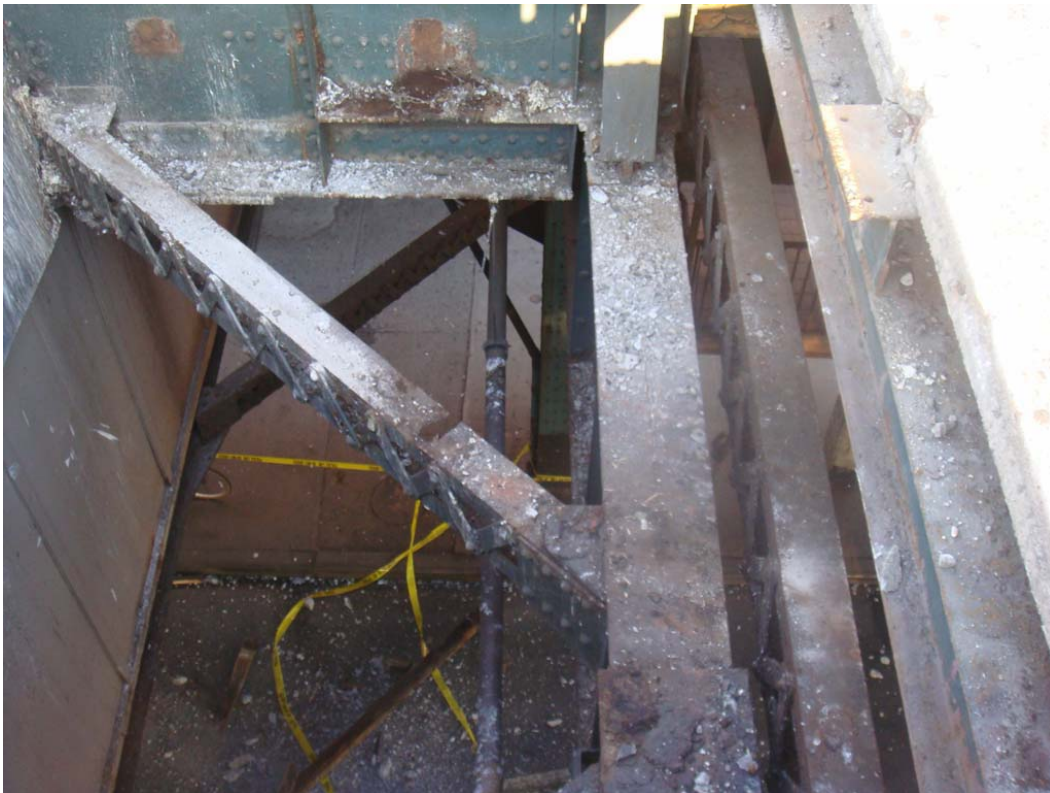
Looking Down at the Street through Platform Hole at the 18 th Avenue Station, May 12, 2009
