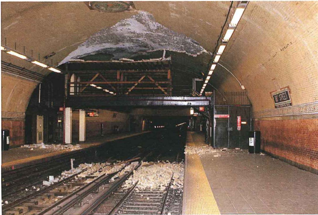
181 st Street Station, Following August 16, 2009 Ceiling Collapse
