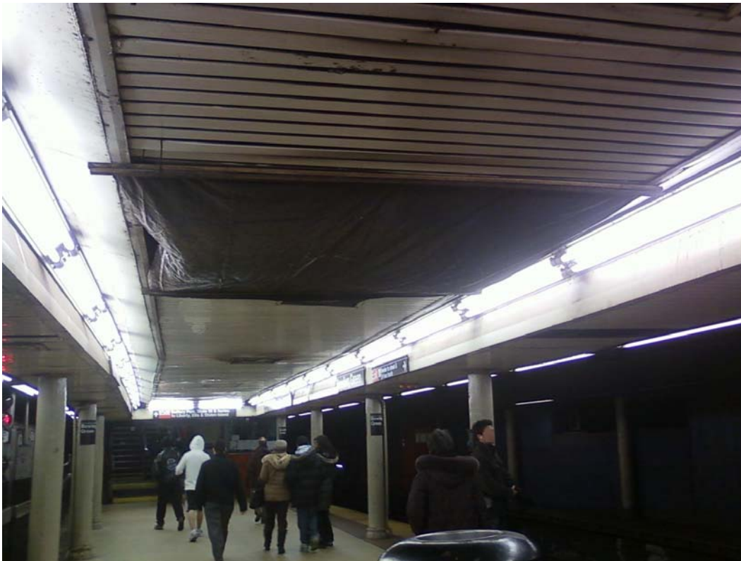
Bowling Green Station with Missing Ceiling Panels, February 17, 2010
