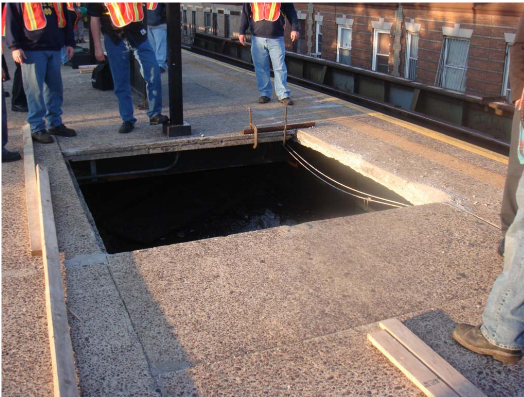
Collapsed Section of 18 th Avenue Station Platform, May 12, 2009
