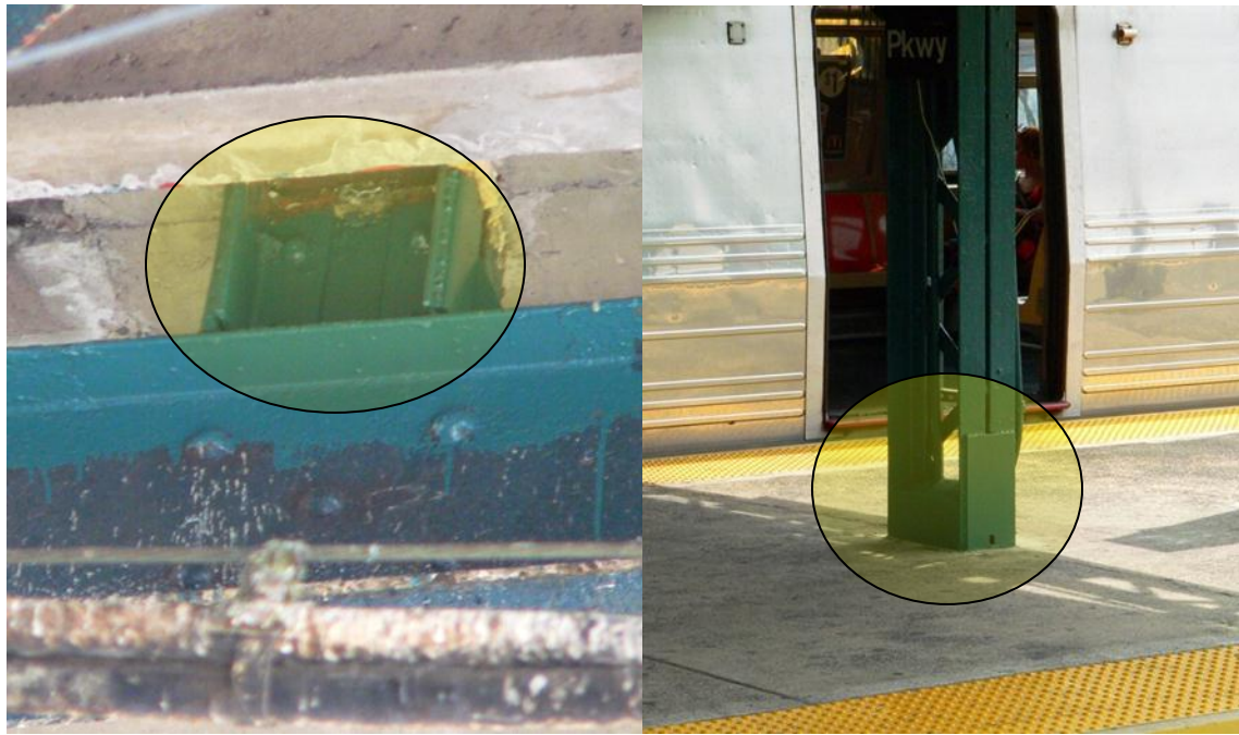
Figure 2: Examples of Repaired Column Bases (View from Below Station on Left; and Side View on Right)
