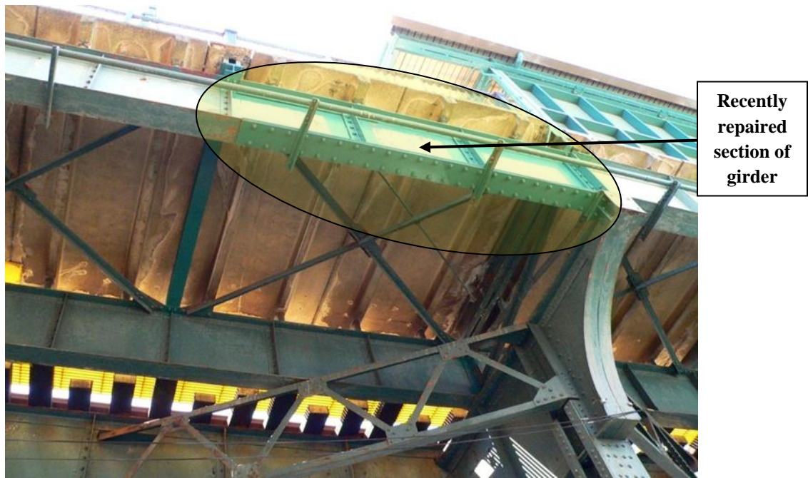
Figure 3: Example of steel girder used to support one of the elevated station platforms at 55 th Street on the D Line, viewed from street level
