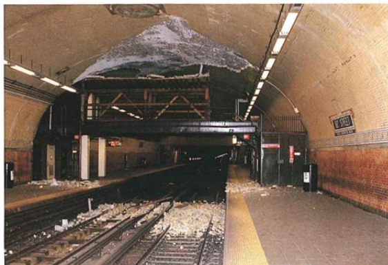
181 st Street Station, Following August 16, 2009 Ceiling Collapse
