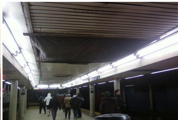
Bowling Green Station with Missing Ceiling Panels, February 17, 2010
