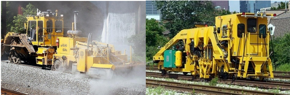
Figure 1: Examples of Track Equipment used by Metro-North. A ballast regulator (left) spreads the stone and distributes it evenly. A ballast tamper (right) is used to pack the ballast under tracks to make the tracks more durable.
