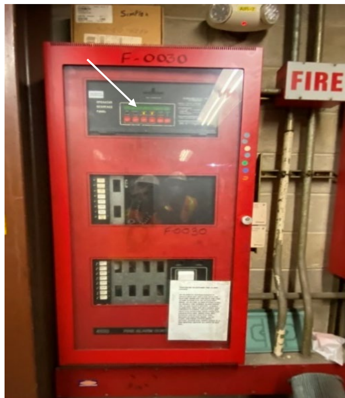
Photo #4: Fire alarm panel indicating both a trouble and a supervisory alarm (top row, yellow lights) at the Coney Island Yard Pneumatic Shop Electrical Room.
