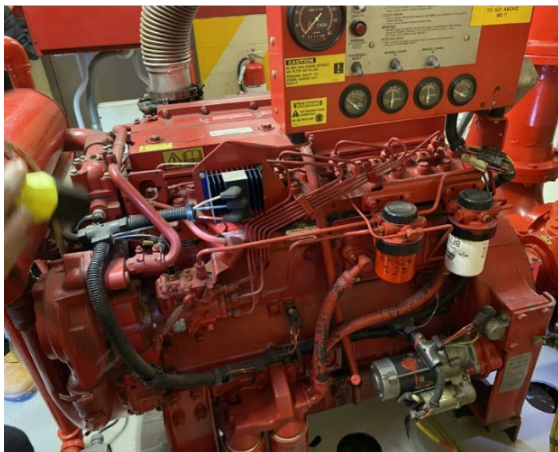
Photo #1: Diesel Fire Pump located in the Overhaul Shop at Coney Island Yard
