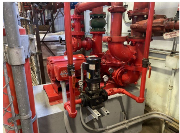
Photo #2: Electric Fire Pump located in Storeroom #1 at 207 th Street Yard
